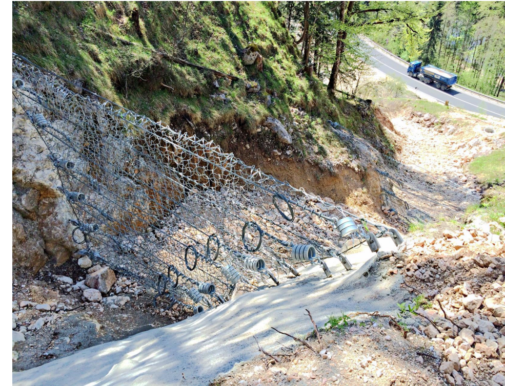
For narrow gullies, no posts are required. The net structure is hung on transverse bearing ropes that are fitted with energy dissipating brake elements. Under ideal circumstances, the gully is bedrock controlled. In unconsolidated material, care must be taken that proper anchoring is available which may sometimes require lateral foundations.
