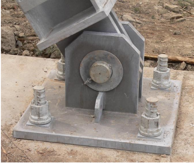
The hinged base plates for the posts and braces are connected to the foundation using short bar anchors or bolts.
