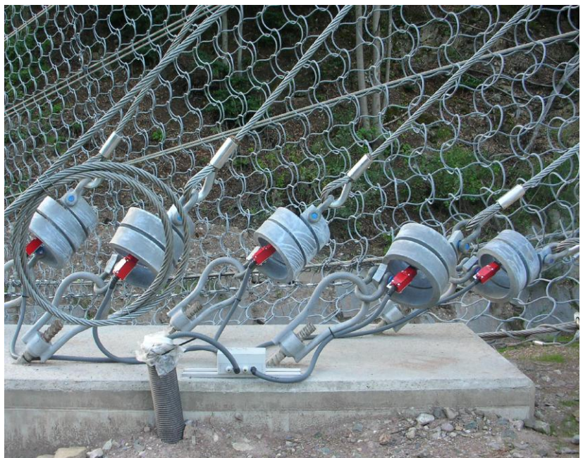
Where there is no bedrock available for anchoring bearing ropes, a concrete foundation with tie-back anchors can be used. Also note, the alarm triggers installed on the brake elements.
