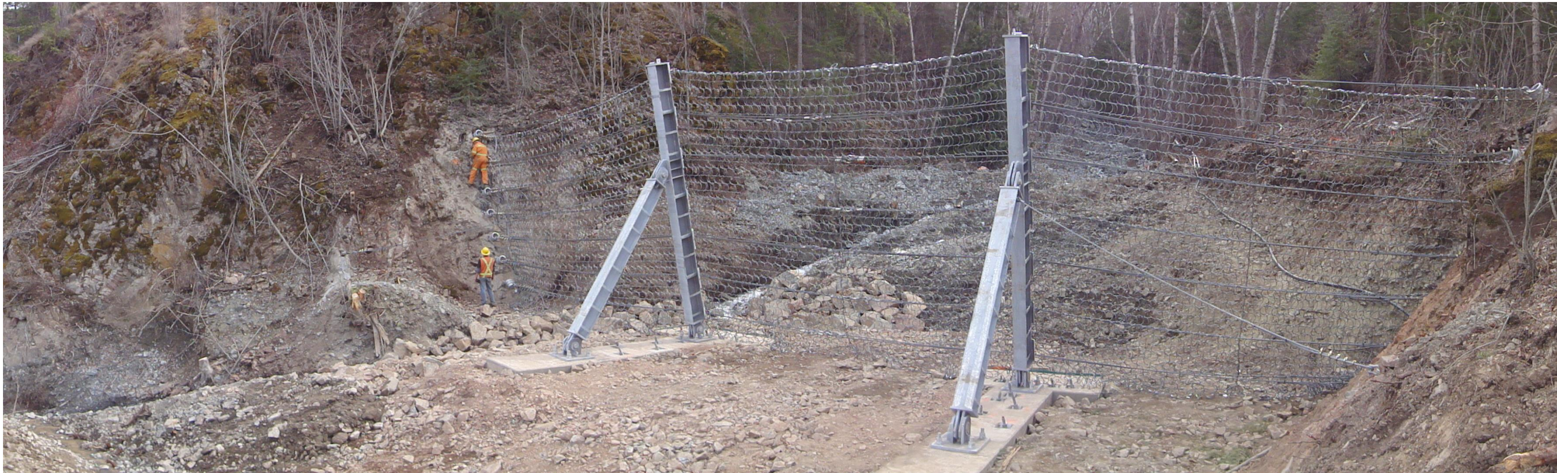
The below structure spans a 30 m gully and stands 6 m tall. It is intended to have a retention capacity of approximately 3000 m 3 .
