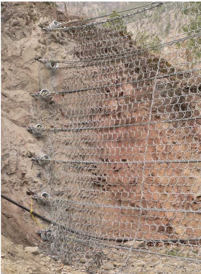
Multiple bearing ropes are used to ensure that the structure can withstand the static loading and dynamic impacts over the entire height of the structure.
