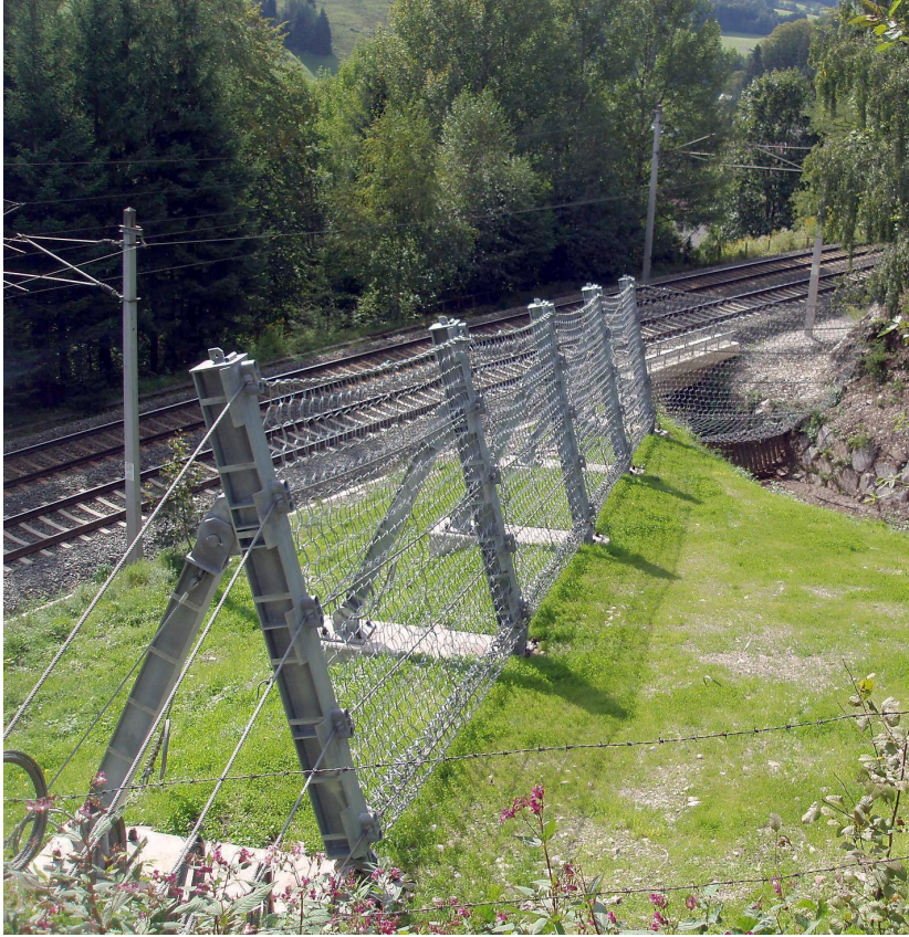
In this example, a 4 m tall debris flow system is used to protect a railway in a partially unconfined deposition area.
