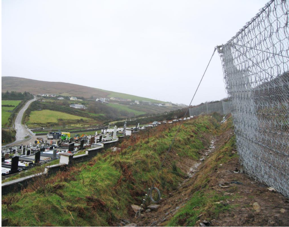
A catchment fence with downslope drainage installed to protect a cemetery from shallow landslides.
