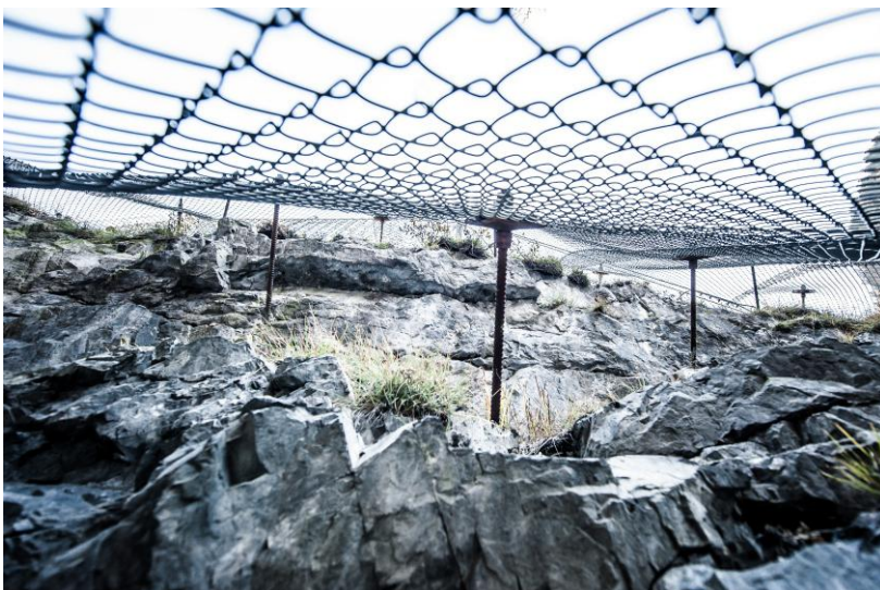
An example of a slope mesh system designed to protect a highway from falling ice that builds up on the slopes during the winter.
