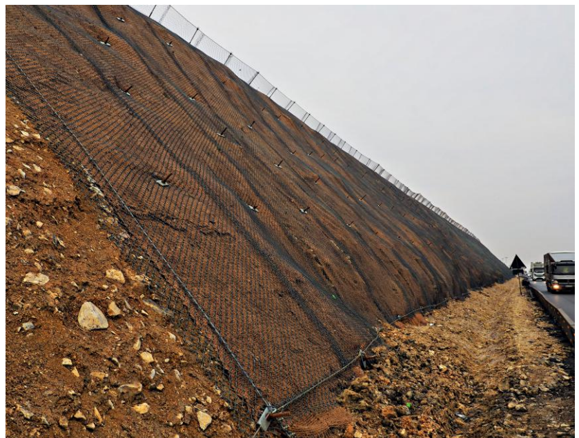
The use of HPN+ in combination with organic mats greatly reduces the lost of fine material and encourages revegetation.
